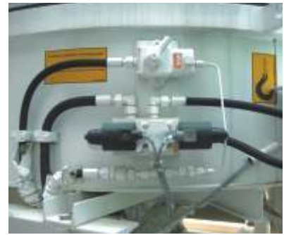
Manual emergency emptying
